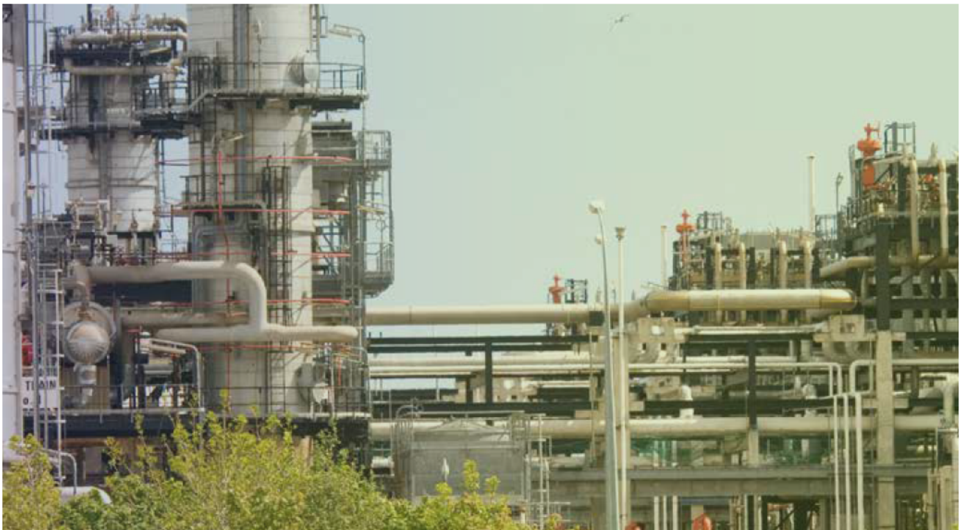
St Fergus Gas Plant, site of future Direct Air Capture project. Credit: North Sea Midstream Partners (NSMP) Limited.
